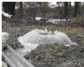
Sewer Manhole Overflow
